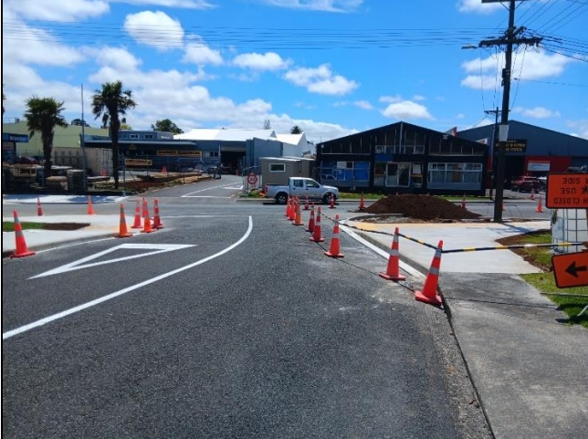
CON22093 Whangarei Urban Traffic Calming - Clark Road and Cambridge Street intersection (Transport Choices) - construction of new kerbs and footpaths connections
