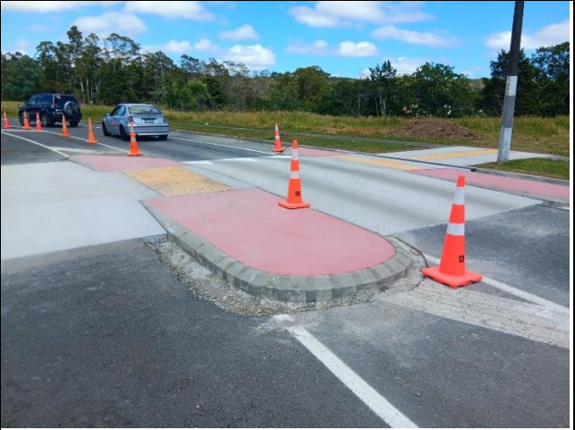
CON22093 Whangarei Urban Traffic Calming - Tauroa Street (Transport Choices) - construction of new concrete courtesy crossing
