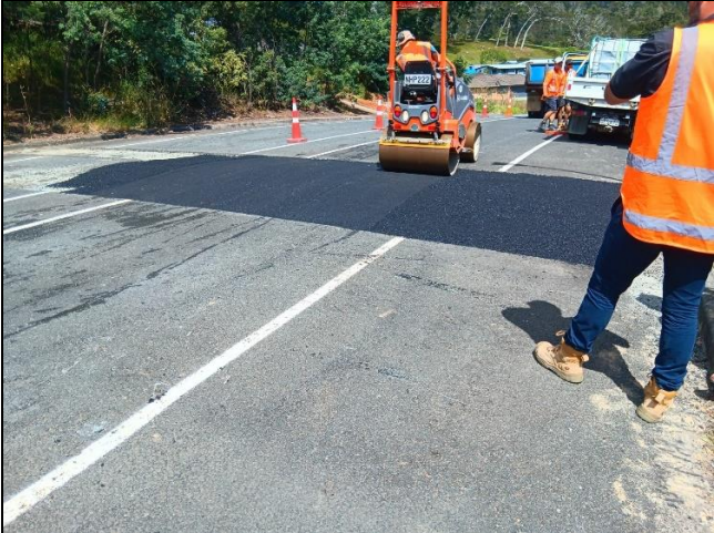
CON22093 Whangarei Urban Traffic Calming - Tauroa Street (Transport Choices) - construction of new asphalt hump
