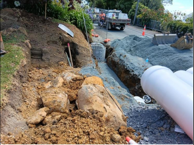
CON24044 Public Transport Improvements (Onerahi) - Old Onerahi Road/Waimahanga Road intersection - Laying renewed stormwater lines and preparing new concrete dish channel
