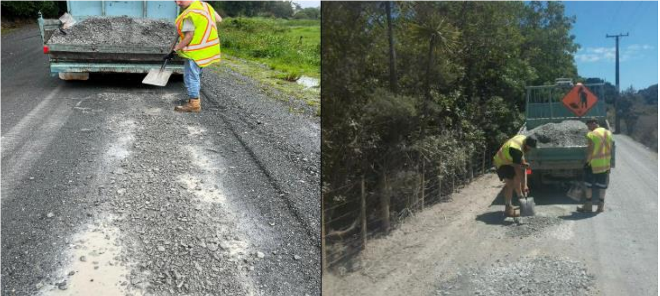
Unsealed Pothole Repairs – Clements Road
