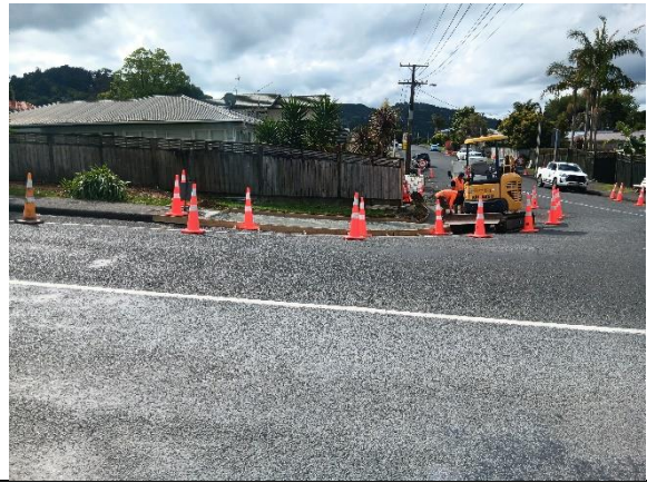
CON22093 Whangarei Urban Traffic Calming – pre pour at Ford Ave intersection with Three Mile Bush Road in Te Kamo (improved pedestrian connectivity/pram crossings)
