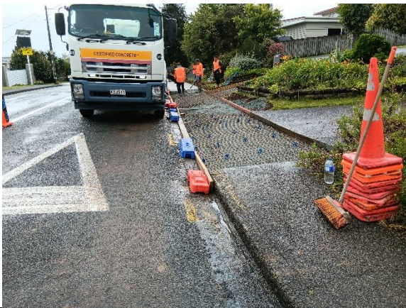
CON22093 Whangarei Urban Traffic Calming – pre pour (footpath renewals) at Three Mile Bush Road roundabout in Te Kamo.
