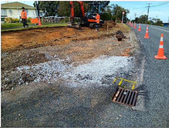
CON24044 PT Improvements – earthworks prep for new/improved recessed concrete bus stop at McKenzie Ave intersection with Church Street, Onerahi
