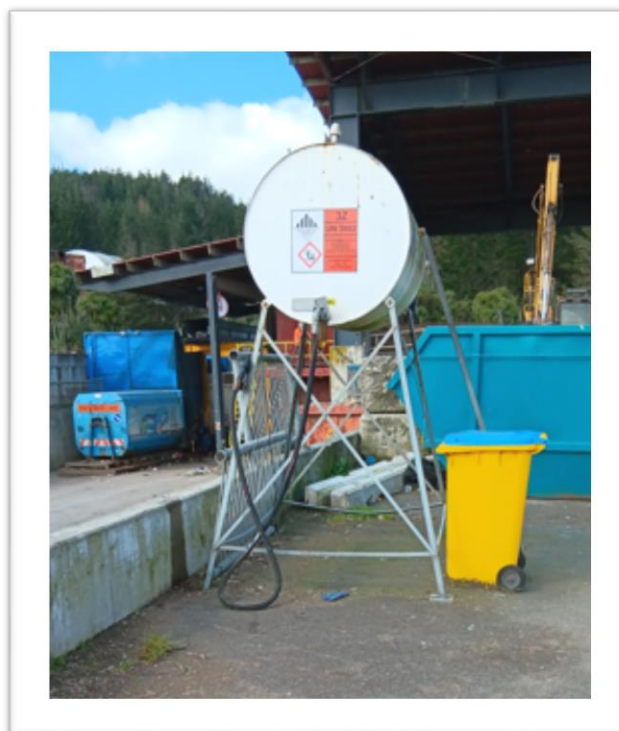
500lt diesel tank.
