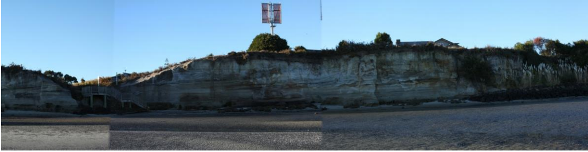
Figure 11: Large eroding cliffs in front of Karoro Road. The navigation beacon can be seen in the middle. The cliffs are replaced by vegetated slopes with coastal protection works immediately to the right of the photograph
