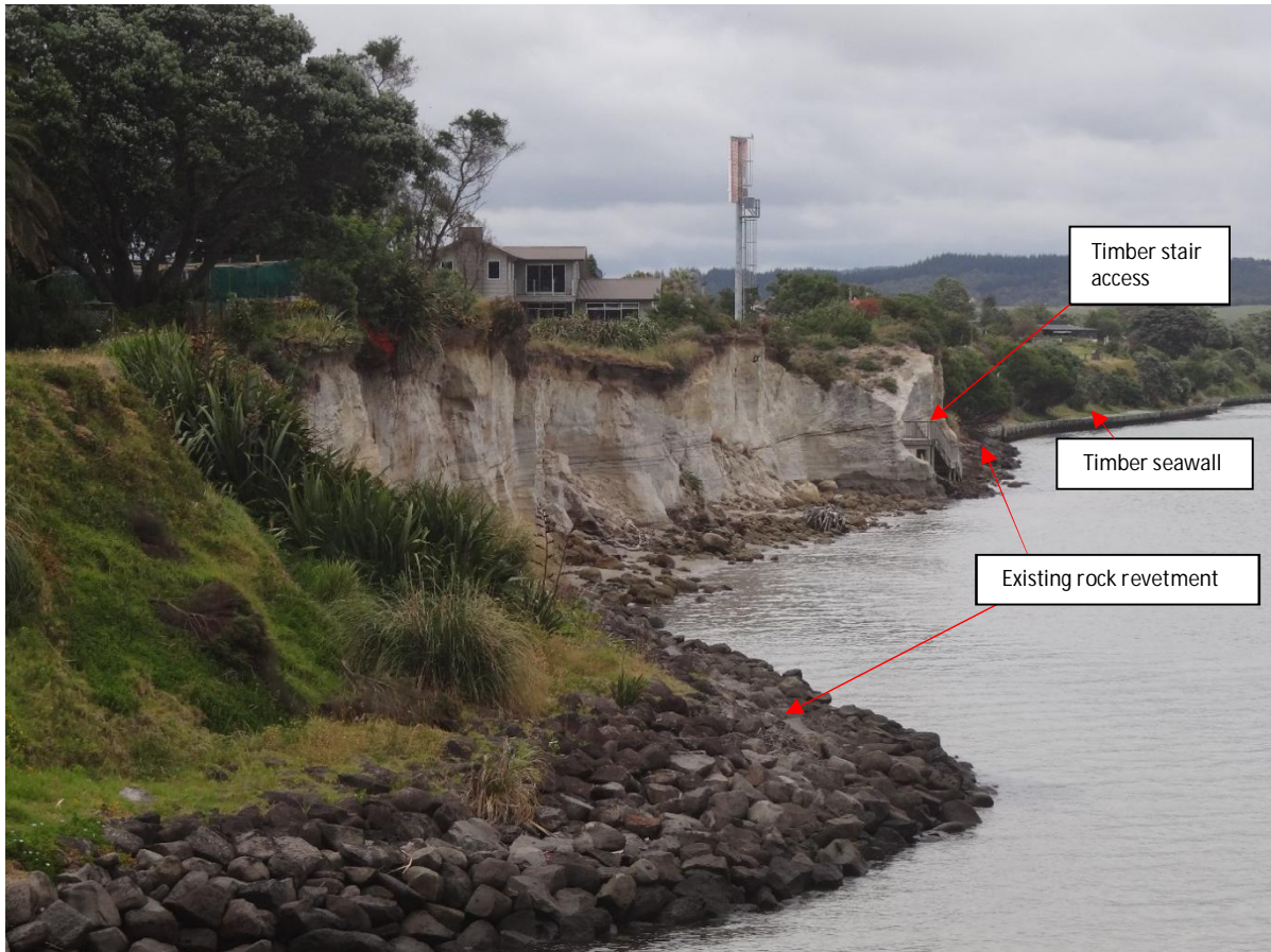
Photograph 5: Looking south along western OTP coastline showing comparison between area that has been armoured by rock and the exposed cliff face at the site. Source: T+T 2014.
