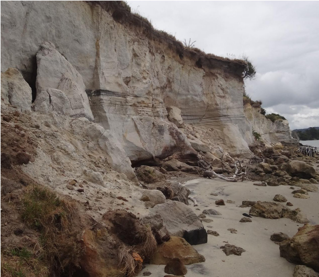
Photograph 4: Northern end of western OTP cliffs showing recent slumping of cliff face. Source T+T 2014.
