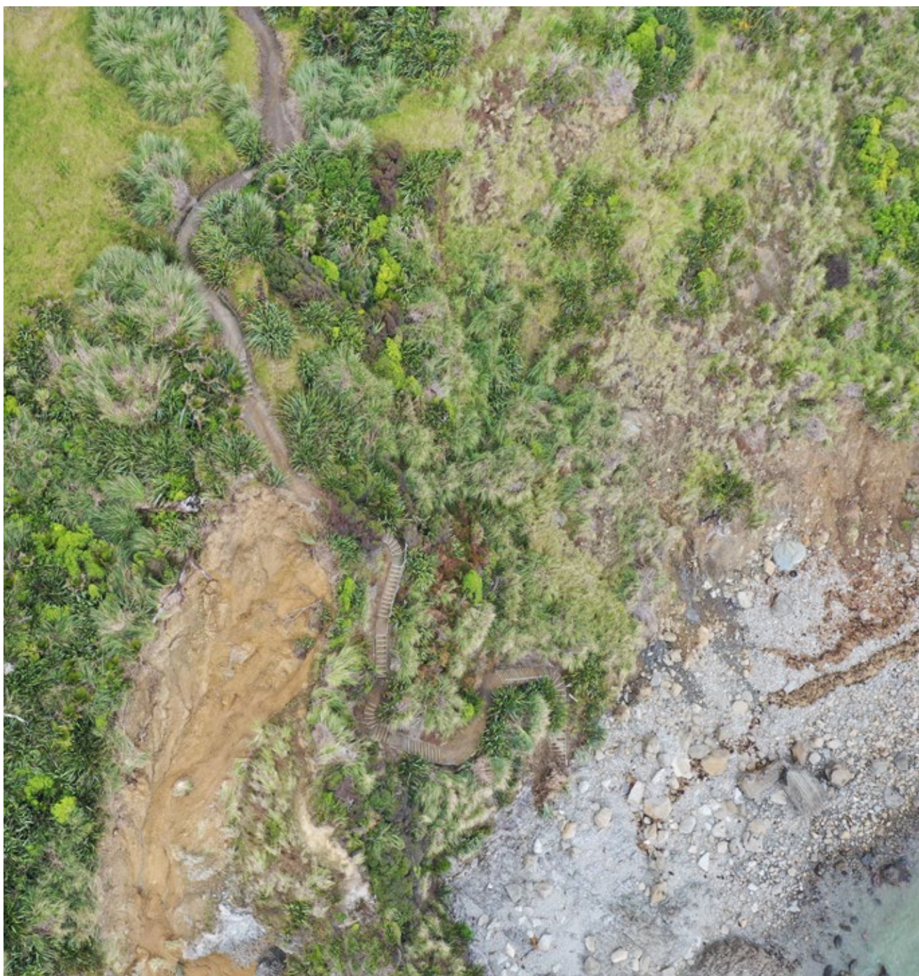
Eroded section of the Mangawhai Walkway
