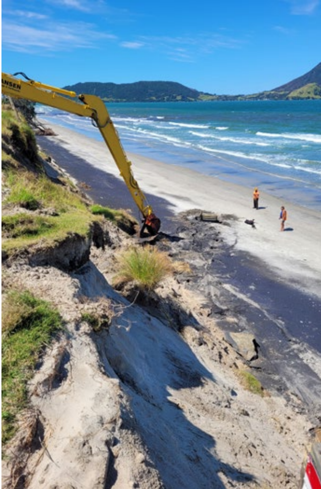
Coastal erosion and remedial works at Uretiti
